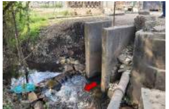
Picture 4-9: Drain carrying dye effluents directly discharges to the outlet drain of 7MLD STP
