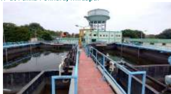
Picture4-3 : 7 MLD STP near Hanuman Mandir, Vindhyachal
