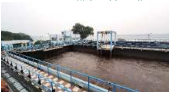
Picture4-2 : 8.5 MLD STP at Bisunderpur, Mirzapur
